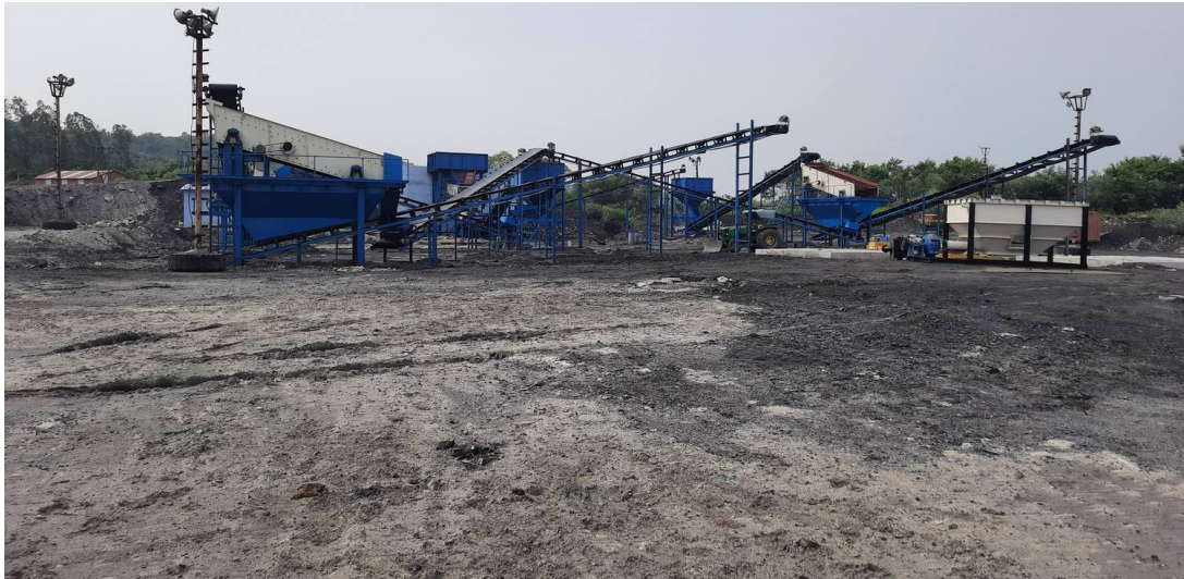
Photo: SREW Projects equipment
